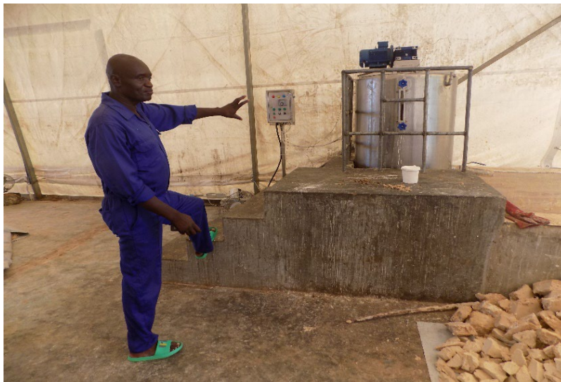
Figure 0-7: Soap factory employee explaining how the boiler works, (Photo by JBN, Nov. 2022)
